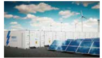
Energy Storage System
