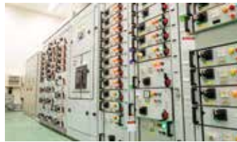
Power Distribution Control
